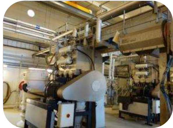
Picture 32: Waste separator
