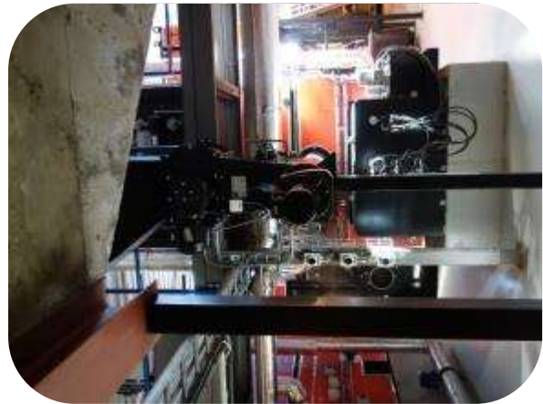
Picture 23: Heating central facilities
