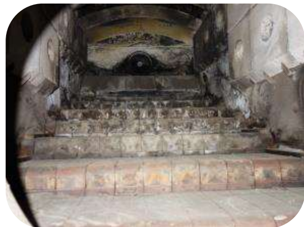
Picture 21: Boiler combustion chamber
