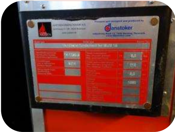
Picture 22: Heating central facilities
