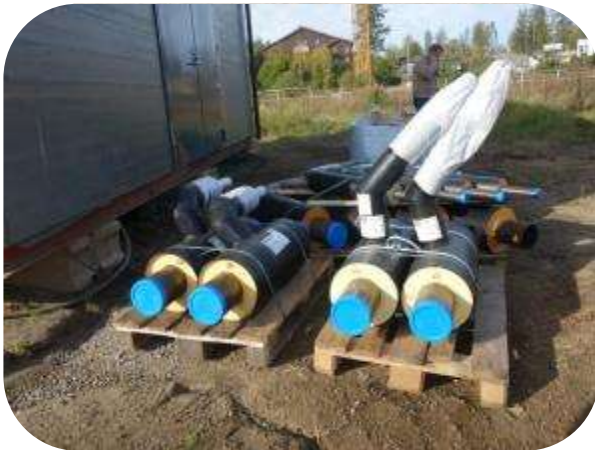
Picture 18: Isolation of heat distribution
