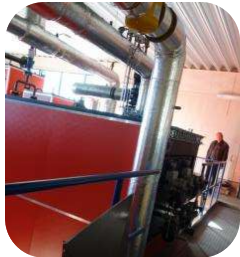
Picture 25: Heating central facilities
