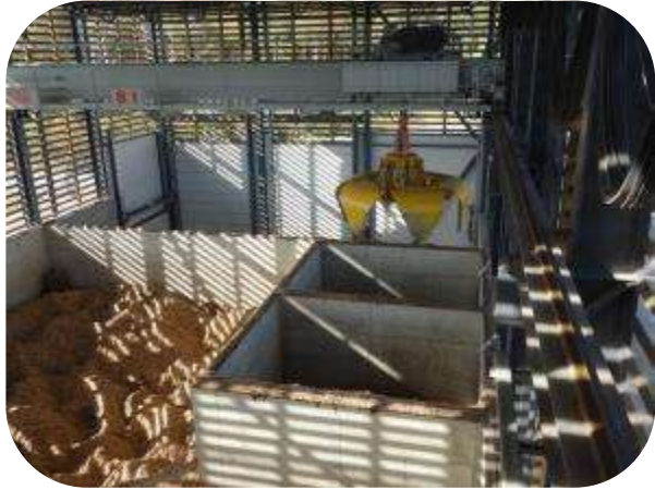
Picture 11: Fuel storage
